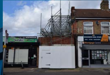
Lot 2 – June Terrace fire damaged house
